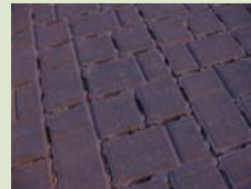
Permeable Pavers Infiltration Practice
