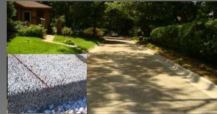
This pervious concrete residential street in Ames, Iowa soaks up rainwater. It looks like regular concrete except that the stones are much larger.
